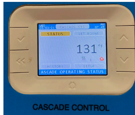
CDB - Cascade Display Board
