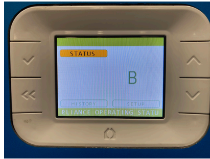
BDB—Boiler Display Board
